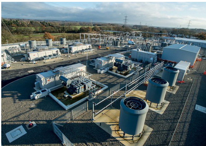
Figure 6: An example of an onshore substation for an offshore wind farm
